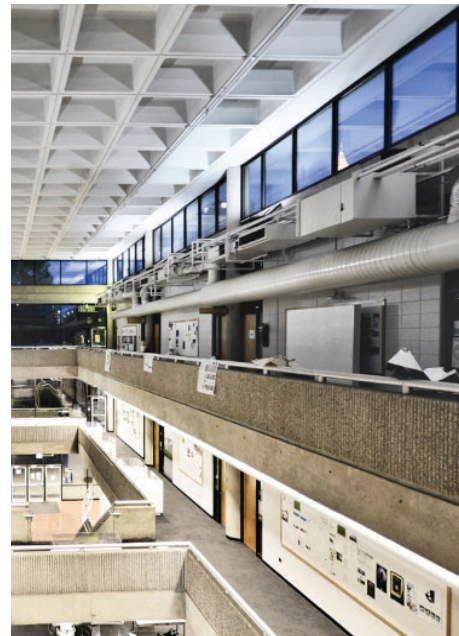
Exposed Utility Pipes // Photo by Shaiba Siddiqui
